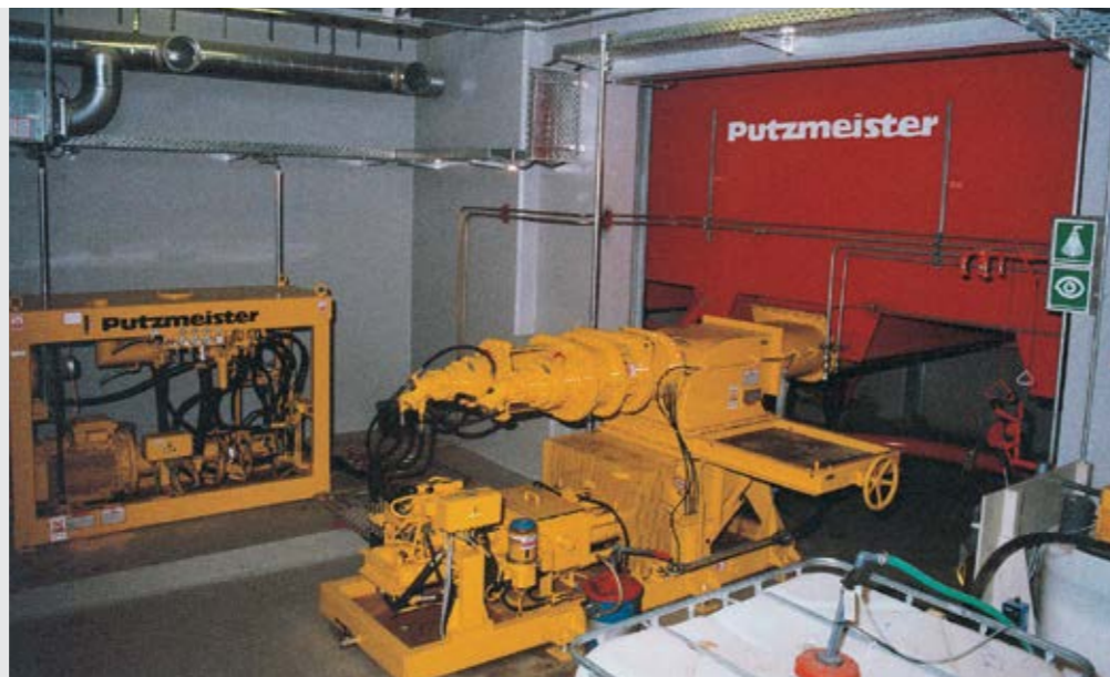
Above: 60 m 3 reception silo with injection pump KOS 540 and power pack HA 45 in the refuse heating and power station at Vestkraft, Copenhagen, Denmark
