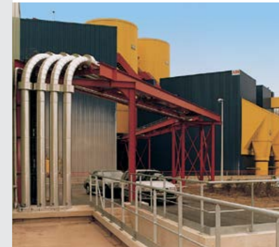
Insulated delivery lines from the reception to the incinerator building
